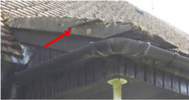
T37 – 7 Mount Pleasant, Wotton-Under-Edge. Front porch, cracking at verge (arrowed)
