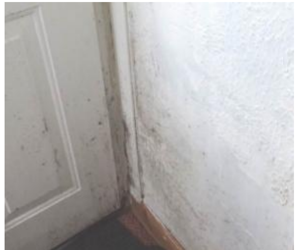
Q10 – 3 Nortonwood, Forest Green, mould in single storey entrance porch
