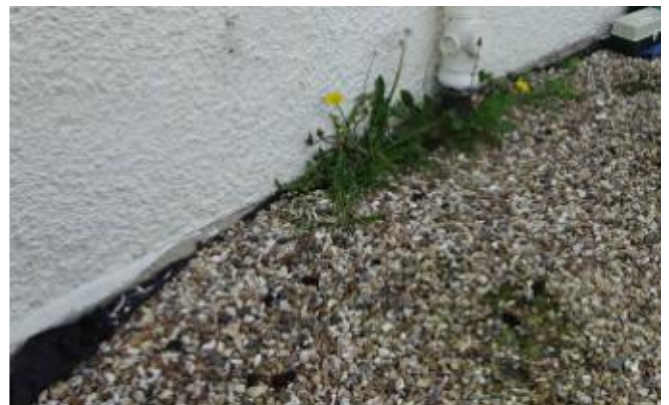
P6 – 14 Mosley Crescent, Cashes Green, ground level at rear too high
