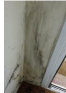
S32 – 51/52 Mankley Road, Leonard Stanley. Mould on external wall at bottom of stairs to first floor flat.
