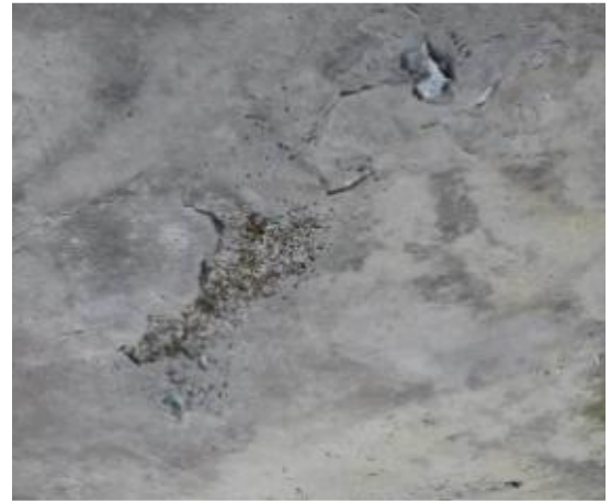
S68 – 31 Victory Road, Whiteshill. Side extension poor finishes to ceiling
