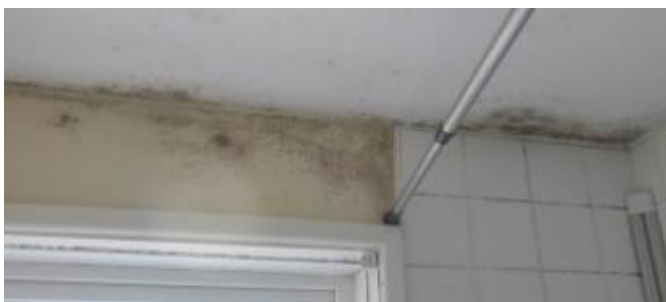
Q11 – 19 Nortonwood, Forest Green, mould in bathroom above window & over bath
