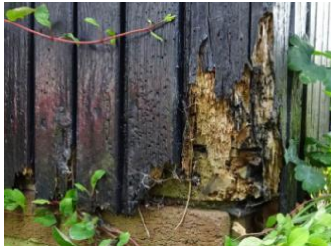
T32 – 3 Mount Pleasant, Wotton-Under-Edge. Front corner, rot & woodworm to outer boards & keel plate.
