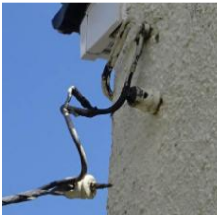
P11 – Overhead power supply fixing at wall, at 14 Hyett Road, Cashes Green
