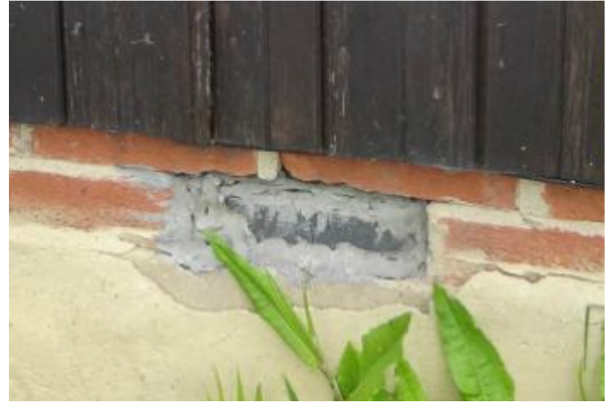
T26 – 6 The Knoll, Uley. Rear, blocked off vent to underfloor void
