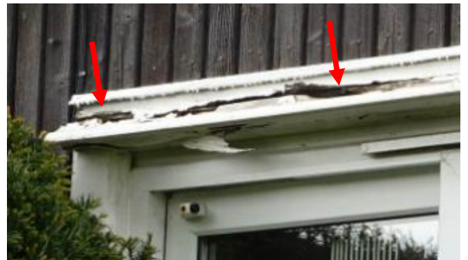
T30 – 8 The Knoll, Uley. Rear, rotten timber architrave above patio doors
