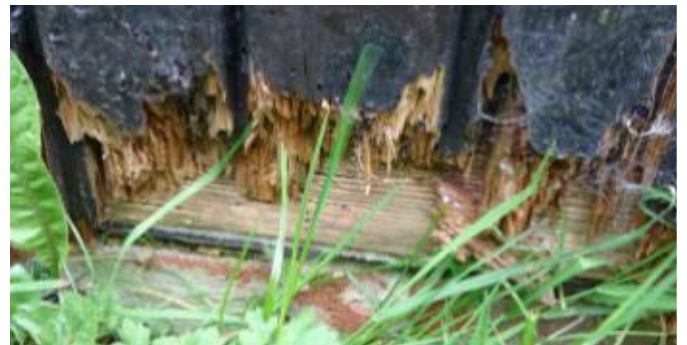
T10 – 32 Barrs Lane, North Nibley. Outbuilding side, rotten timber outer boards & keel plate
