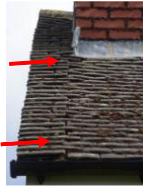
T14 – 3 Bushey Beeches, The Camp. Distortion of roof tiles on line below chimney (arrowed)
