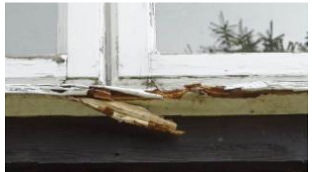
T16 – 3 Bushey Beeches, The Camp. First floor window, rot to window cill
