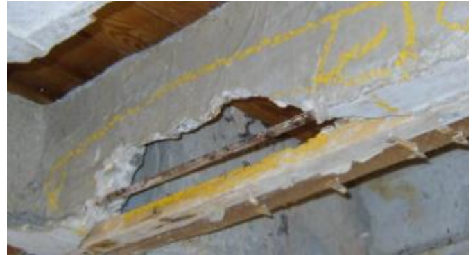
S50 – Typical PRC beam defect (not taken in SDC stock)
