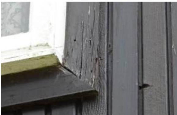
T15 – 3 Bushey Beeches, The Camp. Front first floor window, rot to architrave
