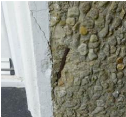
S27 – 56 Lawnside, Forest Green, front spalling to right of front door. Corroded steel & crack
