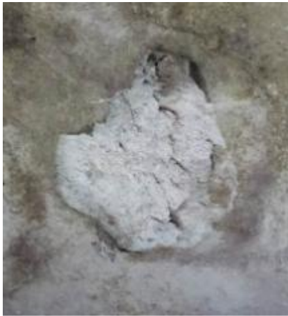
S67 – 31 Victory Road, Whiteshill. Side extension spalling concrete to ceiling
