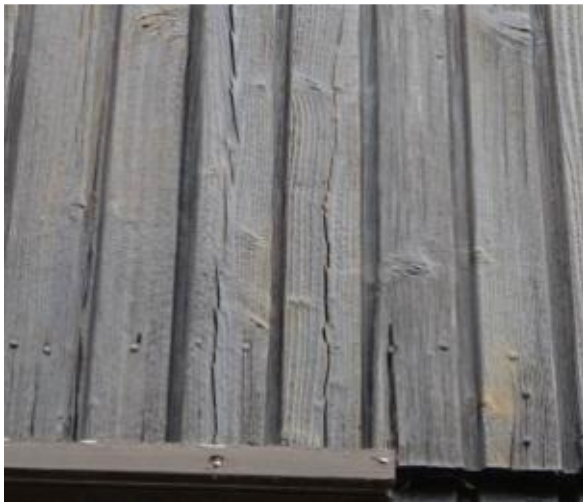
T27 – 6 The Knoll, Uley. Rear, example of rot & split outer boards above patio doors
