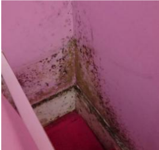
P7 – 14 Mosley Cresnet, Cashes Green, mould in front ground floor room used as bedroom
