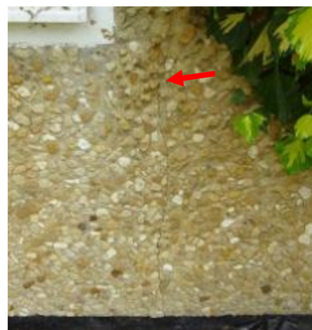
S71 – High Field, crack under front window
