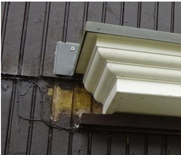
T21 – 6 The Knoll, Uley. Front, replacement canopy leaves untreated timber outer boards
