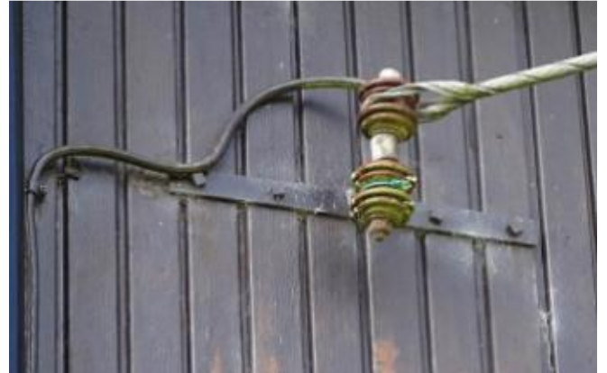
T20 – 3 Bushey Beeches, The Camp. Incoming mains electrics on side elevation
