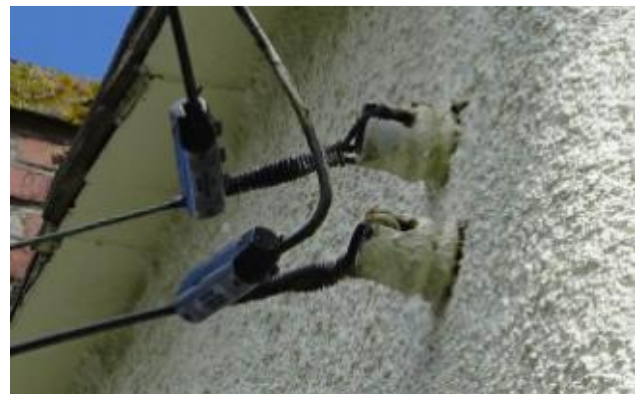
P10 – Overhead power supply fixing at wall, at 10 Kingley Road, Cashes Green
