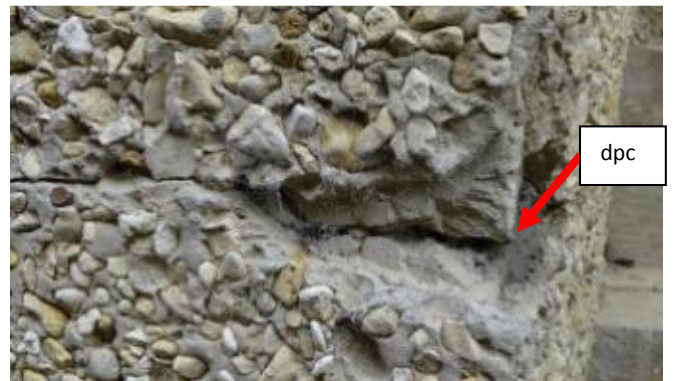
S44 – 6 Upper Park Road, Nailsworth. Side extension, cracking at dpc level detail
