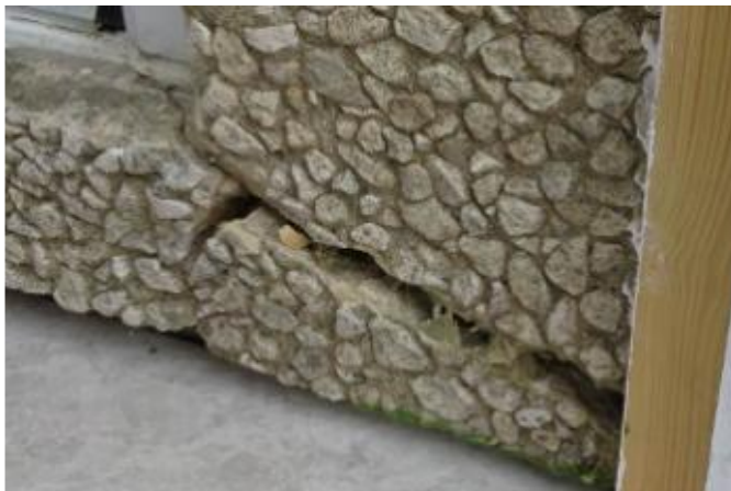
Q9 – 6 Badgers Way, Forest Green, broken panel section to right of front door (within porch)
