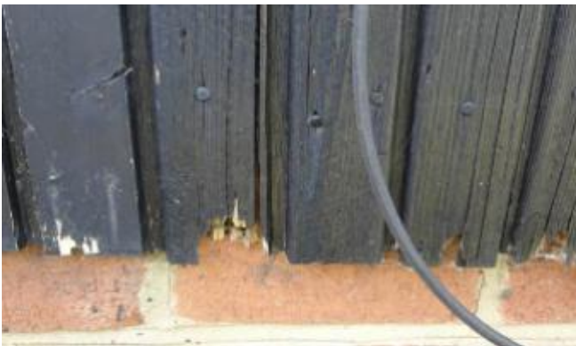
T39 – 7 Mount Pleasant, Wotton-Under-Edge. Rear, rotten outer boards at dpc level
