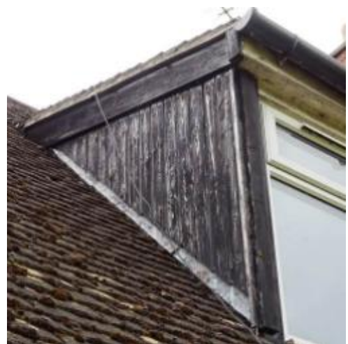
T12 – 32 Barrs Lane, North Nibley. Rear, poor timber to dormer side and architrave
