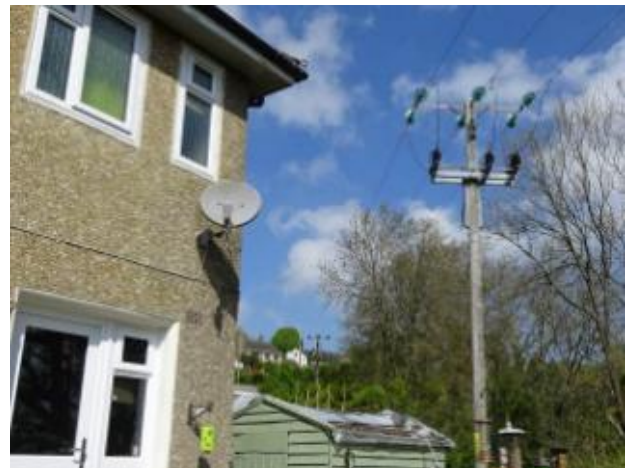
S70 – 26 Victory Road, Whiteshill. Power lines close to the building
