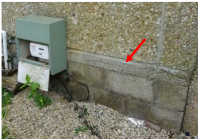
S45 – 6 Upper Park Road, Nailsworth. Rear corner main house. Cast in-situ concrete (arrowed) & blockwork suggests underpinning
