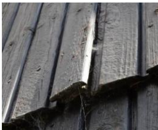
T17 – 3 Bushey Beeches, The Camp. First floor outer boards, board "sprung" due to failed fixing
