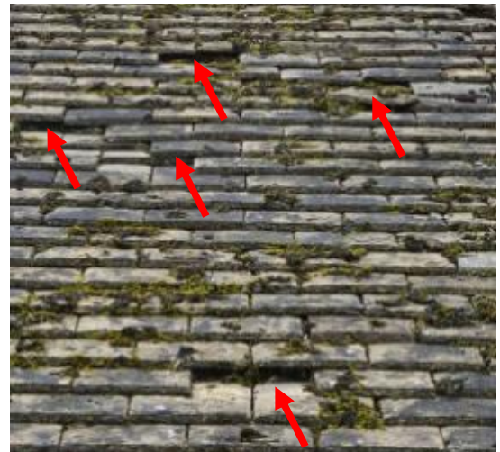
T22 – 6 The Knoll, Uley. Outbuilding front roof, slipped & missing tiles
