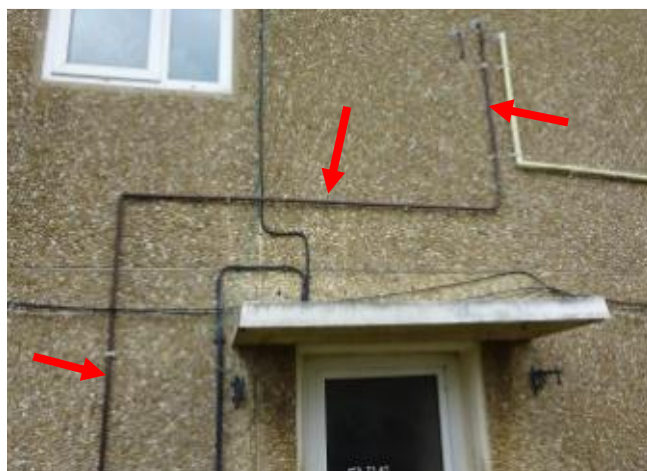
S35 – 51/52 Mankley Road, Leonard Stanley. Gas pipework on external wall
