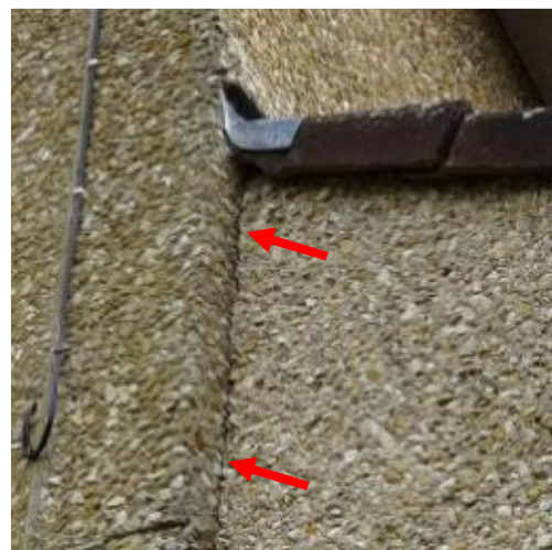
S40 – 6 Upper Park Road, Nailsworth. Cracking at junction of side extension & main house
